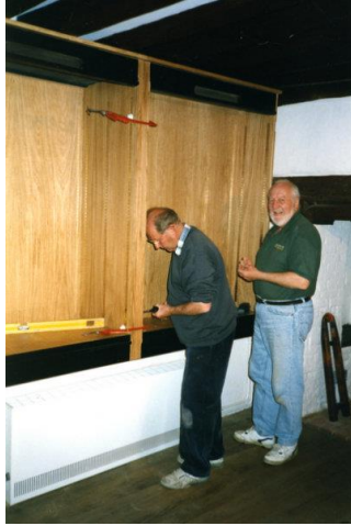
Ken Cooper and Bob Orridge constructing a display cabinet in the Lower Hall, 2000.
